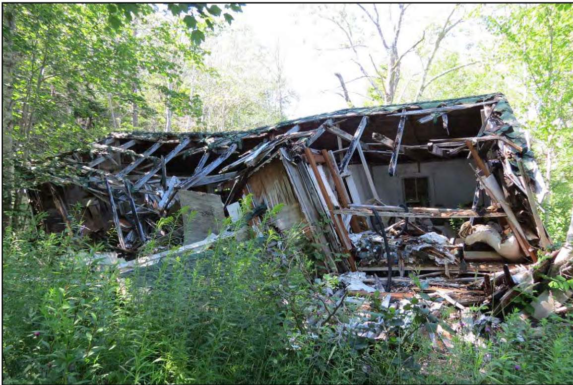
PLATE 21: Abandoned and collapsed cottage along Highway 217; facing north. July 25, 2015.
